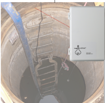
RMC-1000MH Monitoring Unit in Manhole
